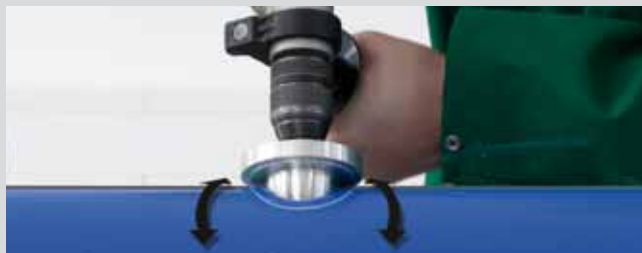
Removal of the oxygen barrier layer from the aquatherm blue pipe or
