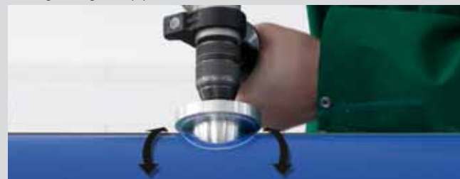
Removal of the oxygen barrier layer from the aquatherm blue pipe of
